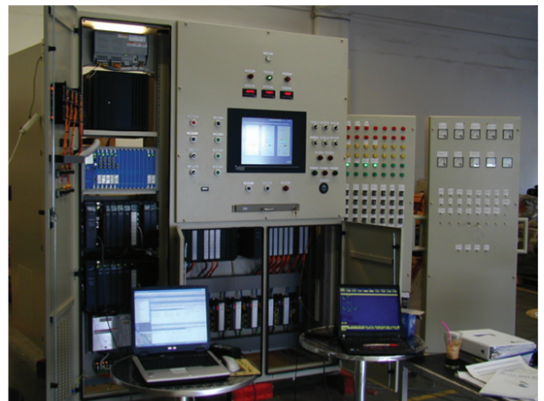
Panel during FAT Tests
